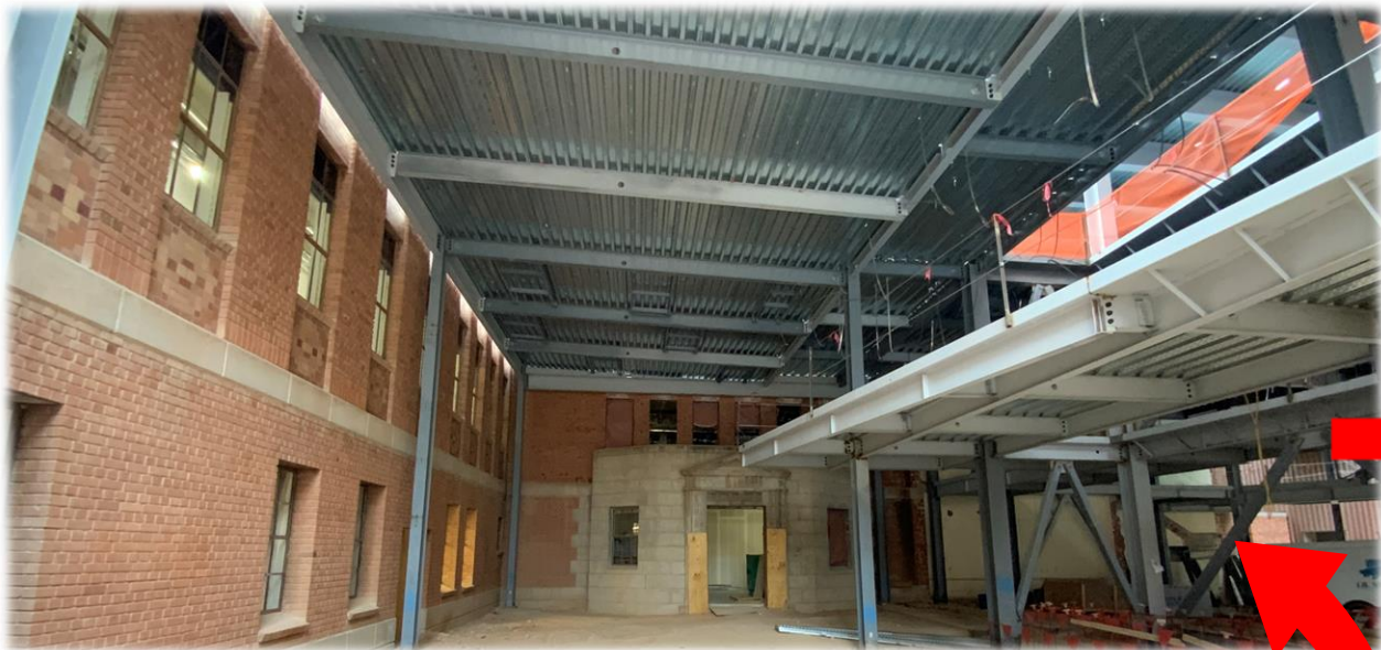
The Commons The new lobby roof deck is on. This space will tie the historic building to the new construction.
